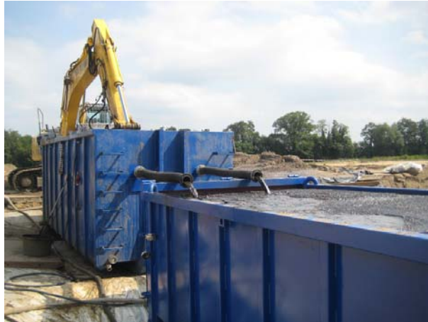
Fig. 8: OSBO® on site soil washing in a special container with downstream multifunctional separation stage.
