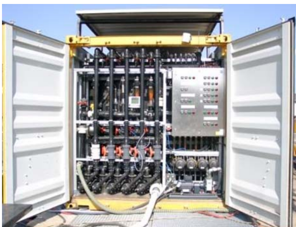
Fig. 11: Biological and oxidative process water treatment plant.
